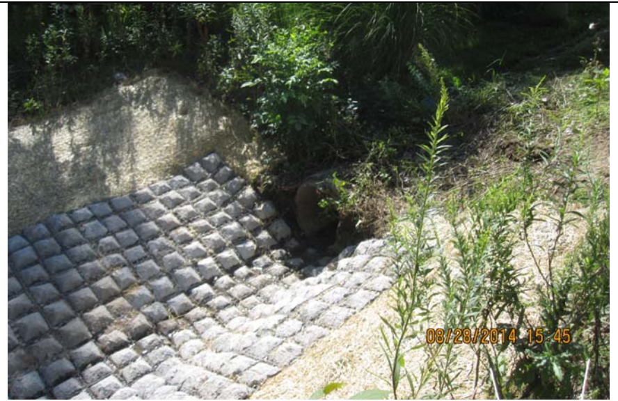
Photo #2: The culverts was originally 50% blocked prior to excavation. Placed flex-a-mat below the culvert outlet for erosion control.
