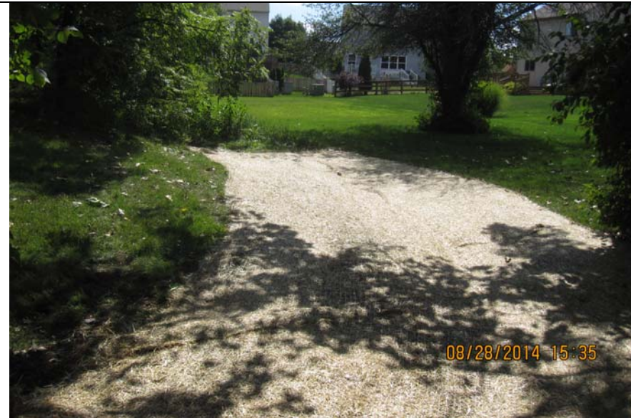
Photo #1: Contractor initially lowered grade a few inches and redirected the flow toward a different drainage swale. Placed straw matting within the finished grades.
